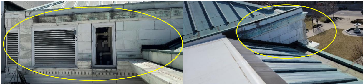
Mortar joints on the northern facing vertical marble panel faces
