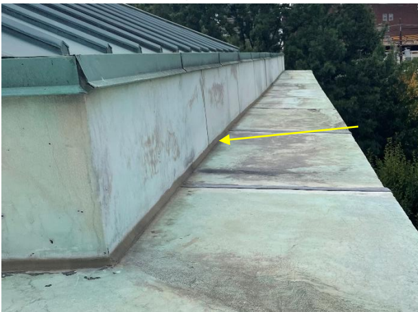
Horizontal joints along the cornice capstone ledges
