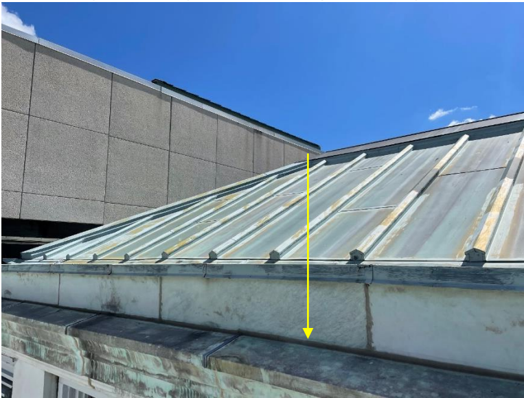
Horizontal joints along the cornice capstone ledges
